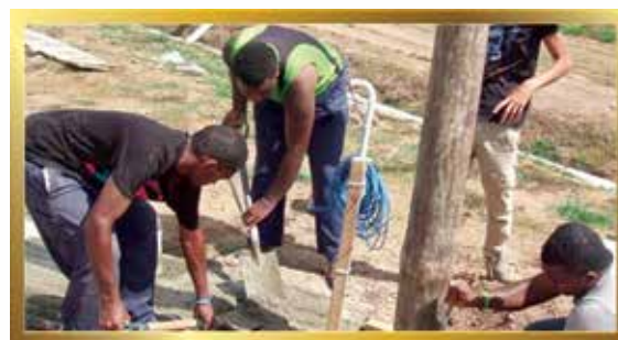
Cabling at Lautoka Women’s Remand Centre
