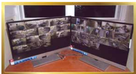
Newly installed Lautoka Remand monitors
