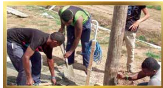
Cabling at Lautoka Women’s Remand Centre
