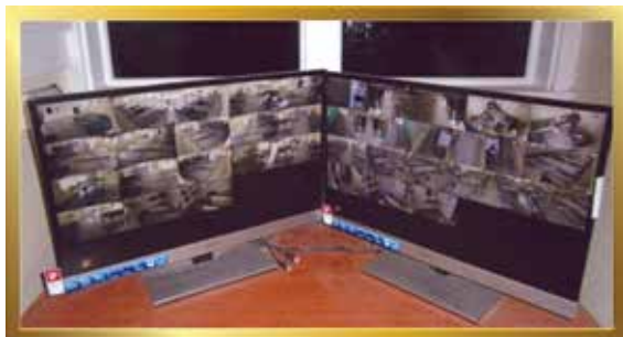
Newly installed Lautoka Remand monitors
